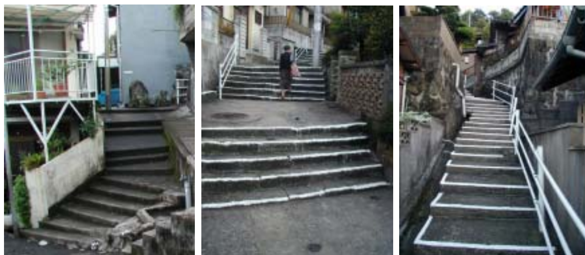
(a) highly irregular stairs
