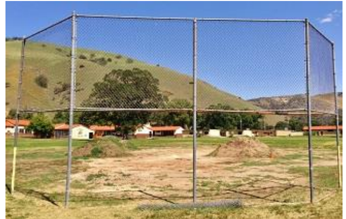
Current field is in the middle of repair; but we need volunteers to sift dirt and we need fencing for foul line poles as we only have the backstop itself.
