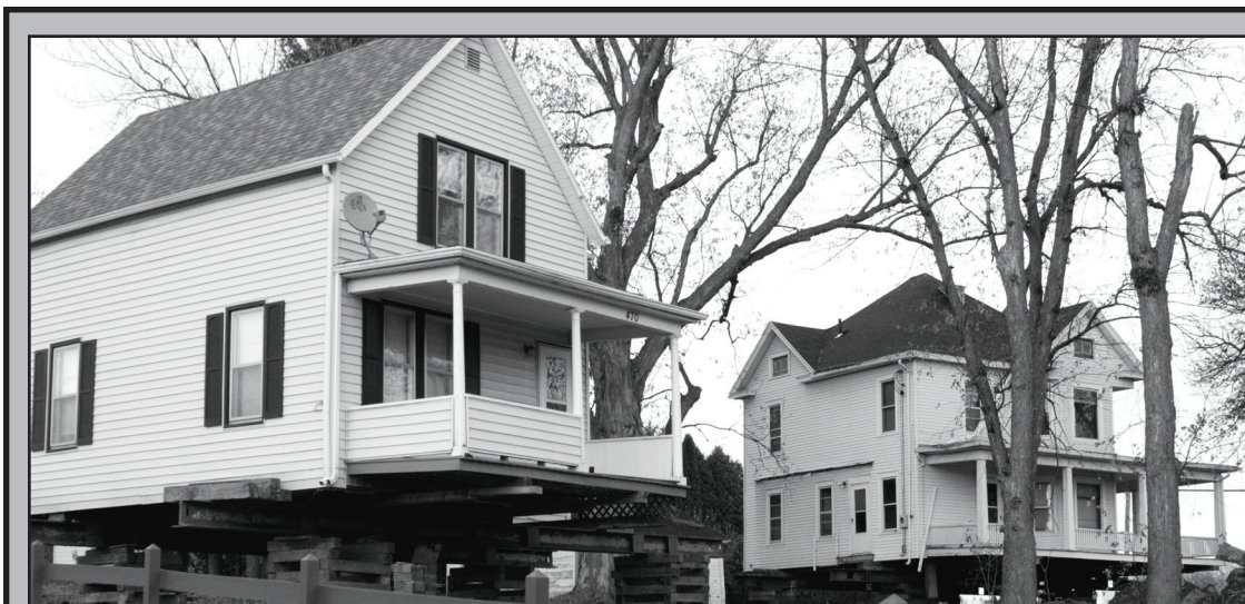
Two houses on Water Street have been raised in preparation for a move. Jodi Krautkramer photos
