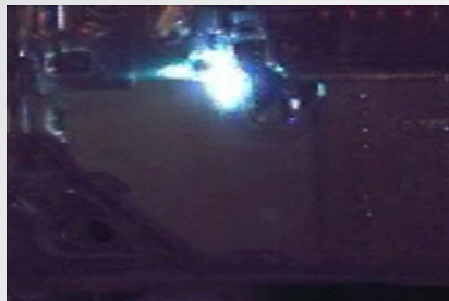
The Fault Current Opens the Solenoid Magnet, Causing The Contacts To Part
