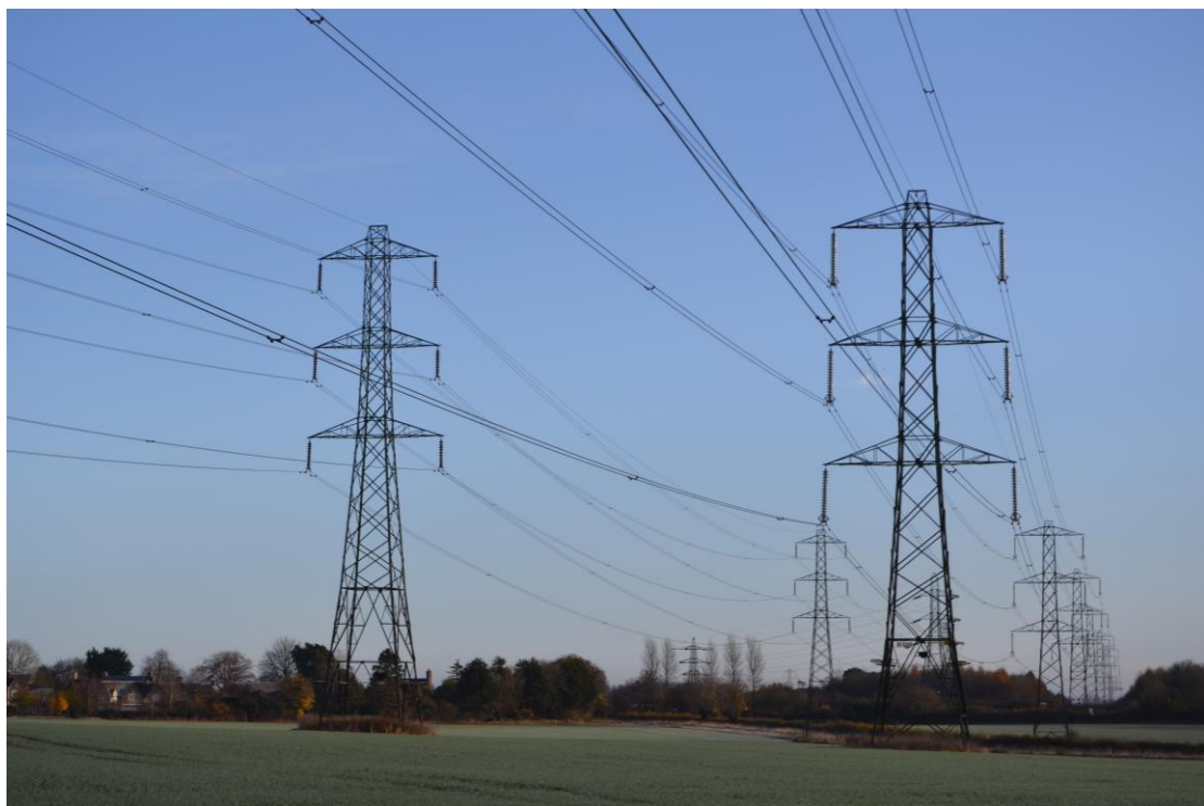
Figure 2 – 132 kV L3 on left. 400 kV L2 lower strung on right.
