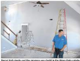
Darryl Hall checks out the progress on a build in the Kings Gate subdivision in Florence.
