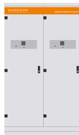
48VDC Power Distribution Panel with Remote Monitoring of DC Voltage and Currents
