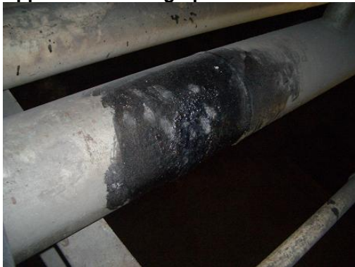
Severe corrosion and leaks on pipe surface
