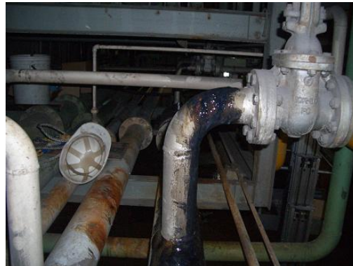
Severe corrosion and leaks on pipe elbow
