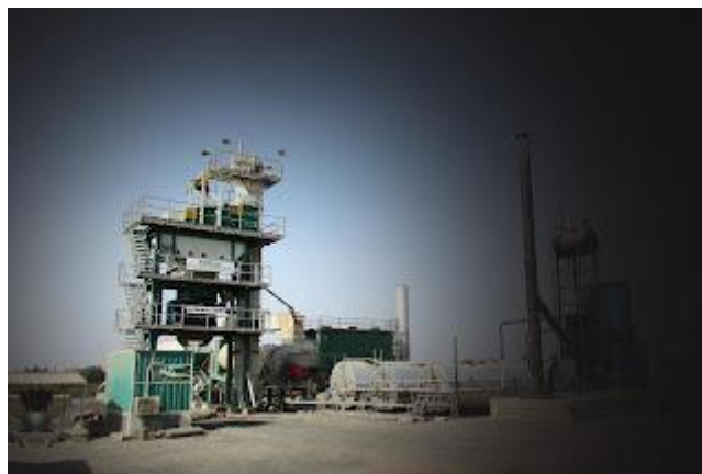
Image:- Asphalt batch mix plant - All Tech Group
